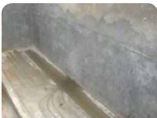
Picture 12: Flooded uninal, Chimteka CBCC
