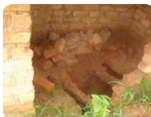
Picture 13: Broken toilets, Kazando CBCC
